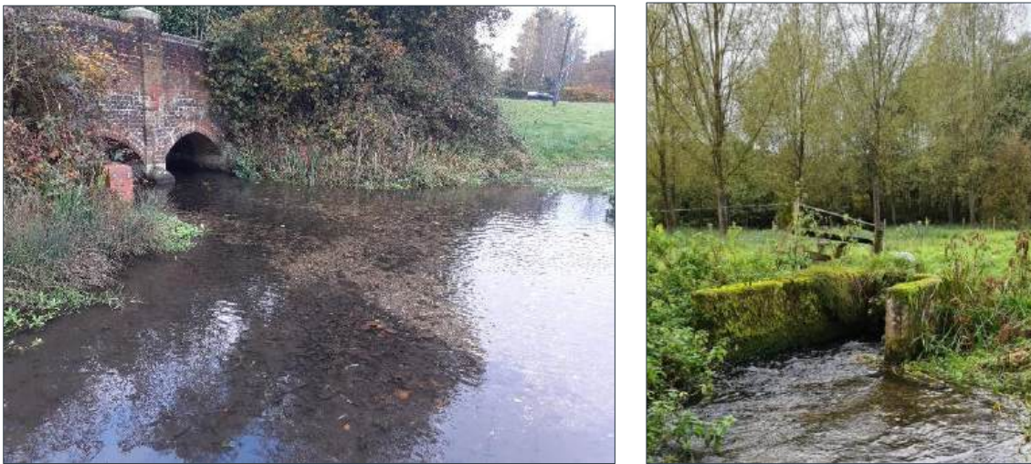
Figure 2.1: Photo of the culvert under Blackwell Hall Lane Road, taken at Subreach 1 (left). Photo of the outfall associated with the Chesham Sewage Treatment Works, taken at Subreach 7 (right).
